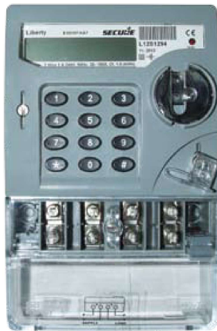
Single phase SABIQ meter
